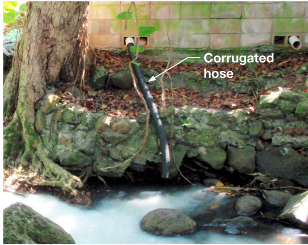
A corrugated hose discharges runoff directly into a stream.
