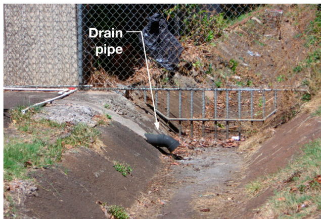
A drain pipe connects runoff from a parking lot directly into a City drainage channel.
