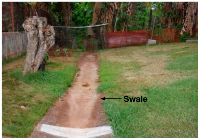
A swale within private property is a private drainage system that typically provides drainage for multiple property owners. Filling, removing, or diverting a drainage system should NOT be done without engineering analysis. These actions change the drainage pattern, which may result in flooding.
