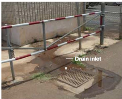
A drain inlet on a private road collects and conveys runoff into the City's storm drainage system.
