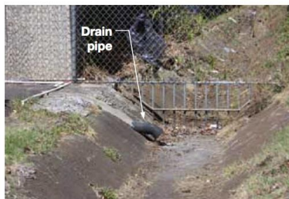
A drain pipe connects runoff from a parking lot directly into a City drainage channel.
