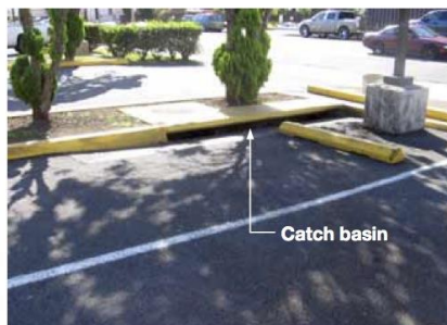
A catch basin in a private parking lot collects and conveys runoff into the City's storm drainage system.
