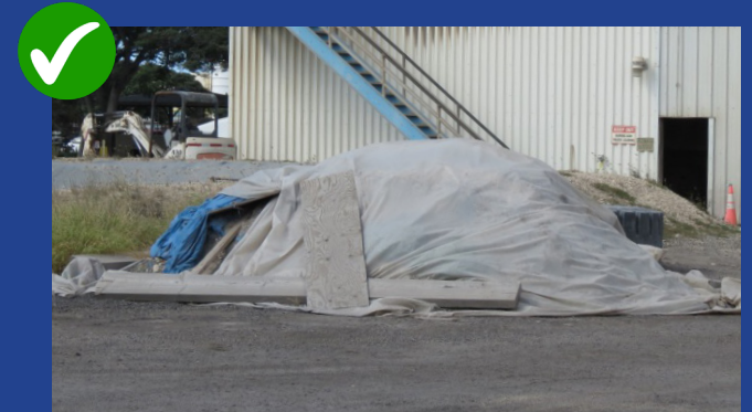
Cover stockpiles and secure covers to protect from rain and high winds.
