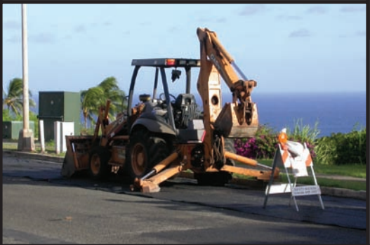
▲ Provide drip pans/material under idle equipment
