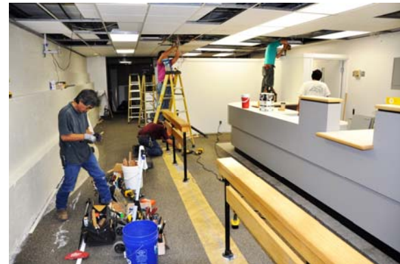
Source: FY 2012 Energy Consumption & Cost Survey and City & County of Honolulu Photobank
