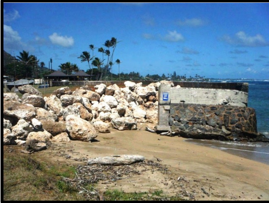
Erosion has caused the seawall along Hau'ula Beach Park to tilt into the ocean.
