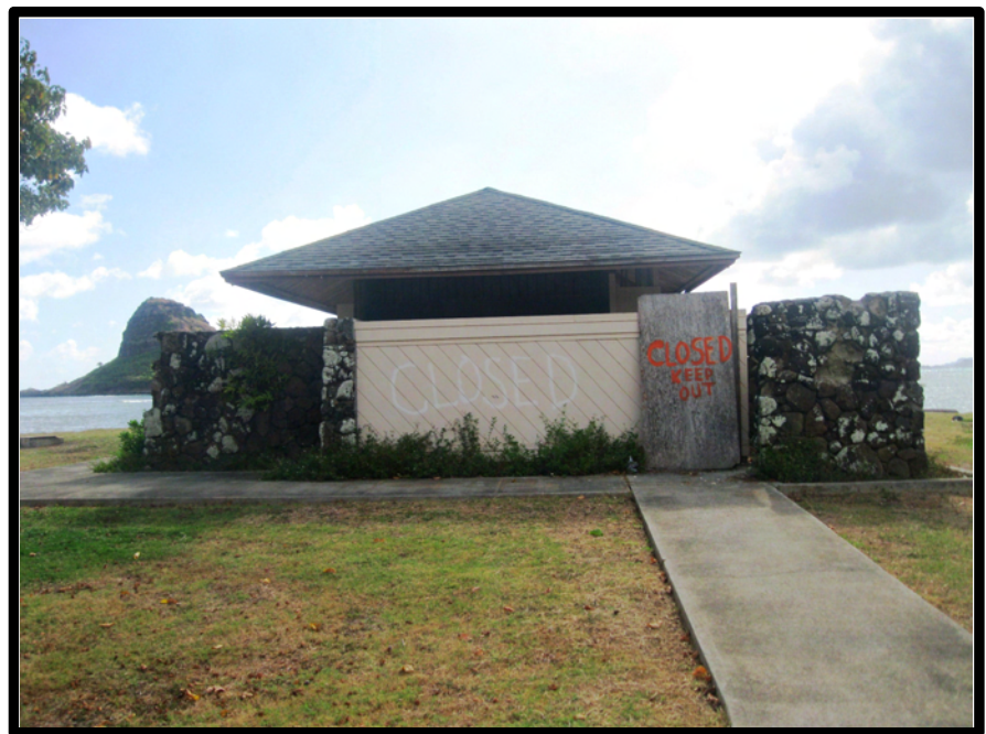
Comfort Station No. 3 at Kualoa Regional Park was condemned in 2005. As a result, 16 campsites in close proximity were also shut down.
