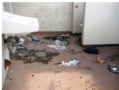
Condemned comfort station is still accessible and used at Kualoa Regional Park
