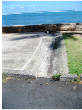
This drainage way diverts runoff from the parking lot directly into the ocean at Swanzy Beach Park
