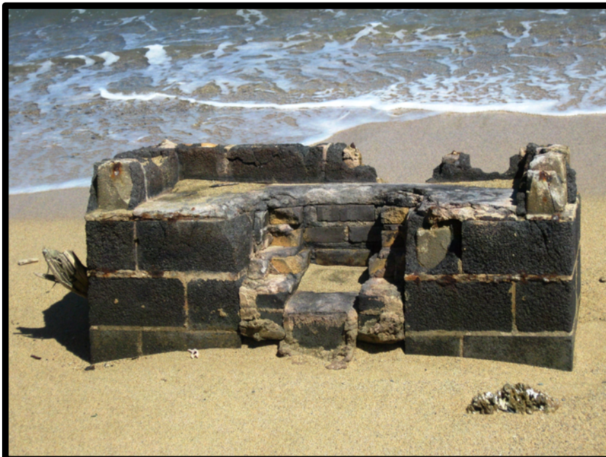
This barbeque pit has fallen onto the shoreline at Hau'ula Beach Park and creates a safety hazard for campers and beachgoers.
