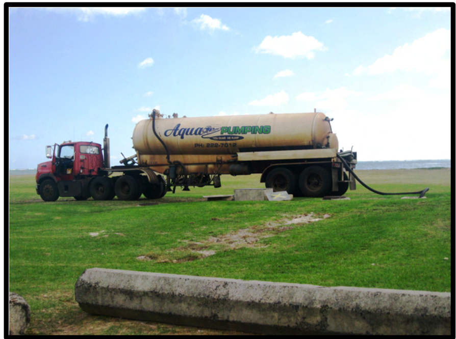
A tanker is seen pumping sewage at Kualoa Regional Park. The city spends about $8,722 per month for trucks to pump wastewater from comfort station tanks.
