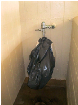
Inoperable, vandalized urinal at Bellows Beach Park
