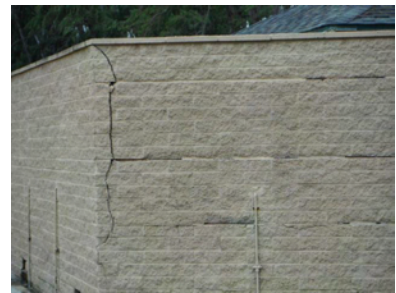
Numerous cracks can be found in restroom walls at Waimanalo Bay Beach Park
