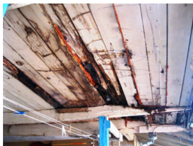
Termite-eaten ceiling at Kualoa Regional Park
