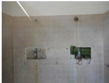
Missing shower tiles and mold at Kalaeloa Beach Park
