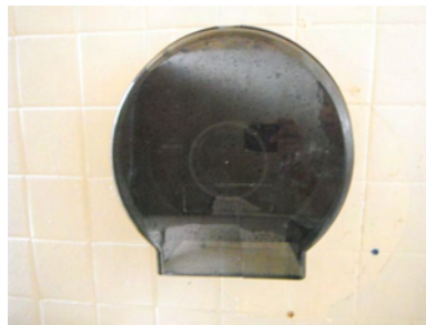
Lack of toilet tissue at Waimanalo Bay Beach Park
