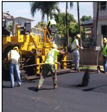
A road repair crew conducts maintenance work on Kilaha Street in Ewa Beach.
