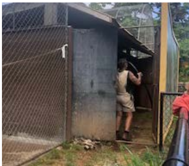
Overgrowth in exhibit; rotting wooden door
