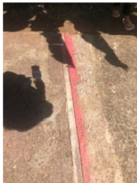
Marked, cracked, lifted sidewalk
