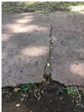
Cracked and lifted sidewalk
