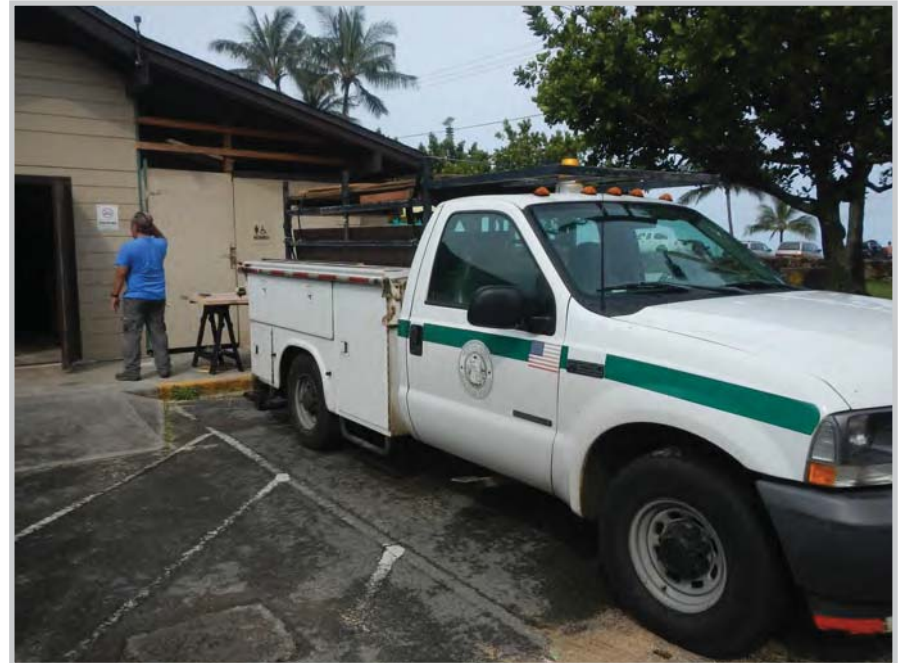
A carpenter with the Maintenance Support Services makes upgrades to the comfort stations at Sunset Beach park, in conjunction with Mayor Caldwell’s Kākou for Parks initiative.
