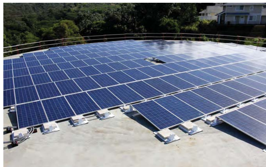
Energy Savings Performance Contract Solar Panels
